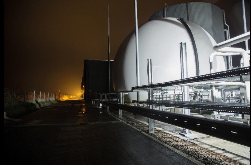
Anaerobic Digestion Plant 2017
